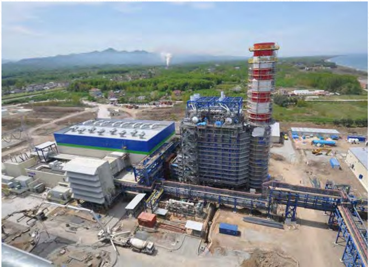
OMV GAS - SAMSUN CONTRACTING AUTHORITY: OMV AUSTRIA, METKA
